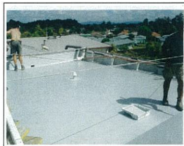
Hamilton Roof—Meridian Energy
